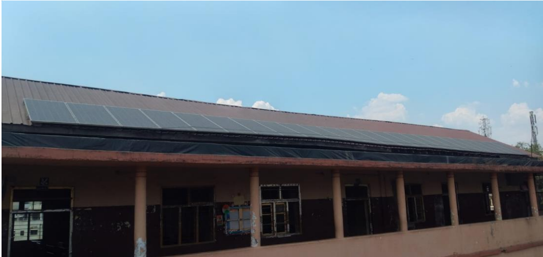
Solar energy Plant
